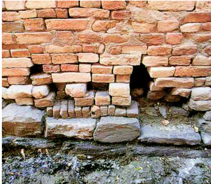
Figure 2.16: Impact on the foundations by 'moto ondosso' (Brighenti et al., 2003, Source: INSULA SpA)
