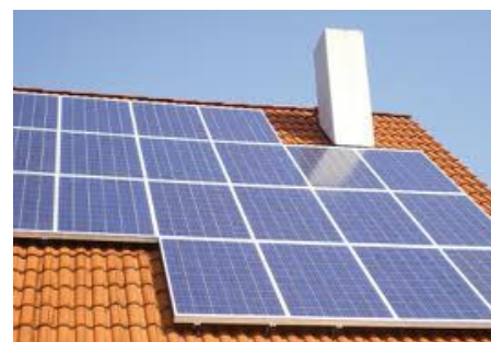
Figure 9: Solar cells on roof, © Köbernik Energietechnik
