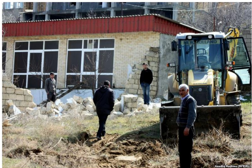
Figure 6: Azersu demolishes dachas (bottom) that were illegally constructed on or within the restricted zone around their pipelines (top).
