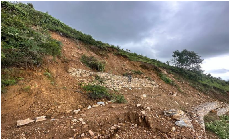
Photograph 3: Debris flow at Nagi dada showing failure of mitigation measure
