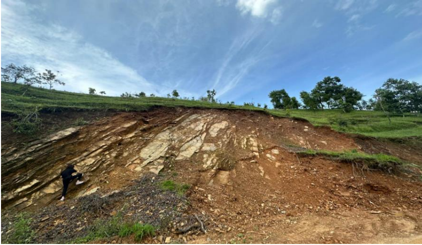
Photograph 4: Landslide due to road cutting in the study area.
