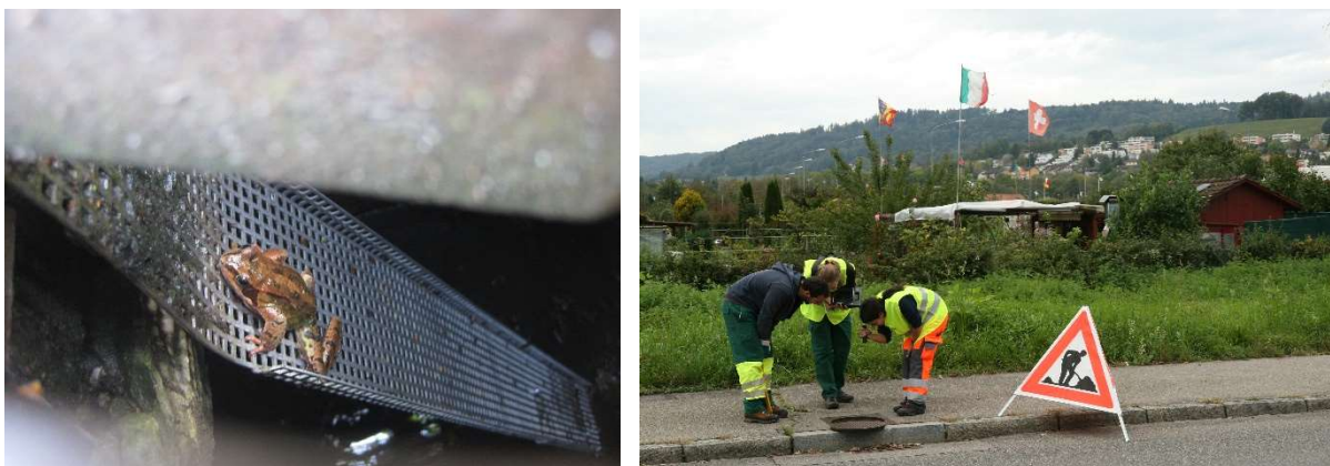
FIGURE 1: LEFT PICTURE: COMMON FROG CLIMBING OUT OF THE GULLY POT USING AN AMPHIBIAN LADDER, RIGHT PICTURE: MONITORING OF GULLY POTS IN ZÜRICH.
